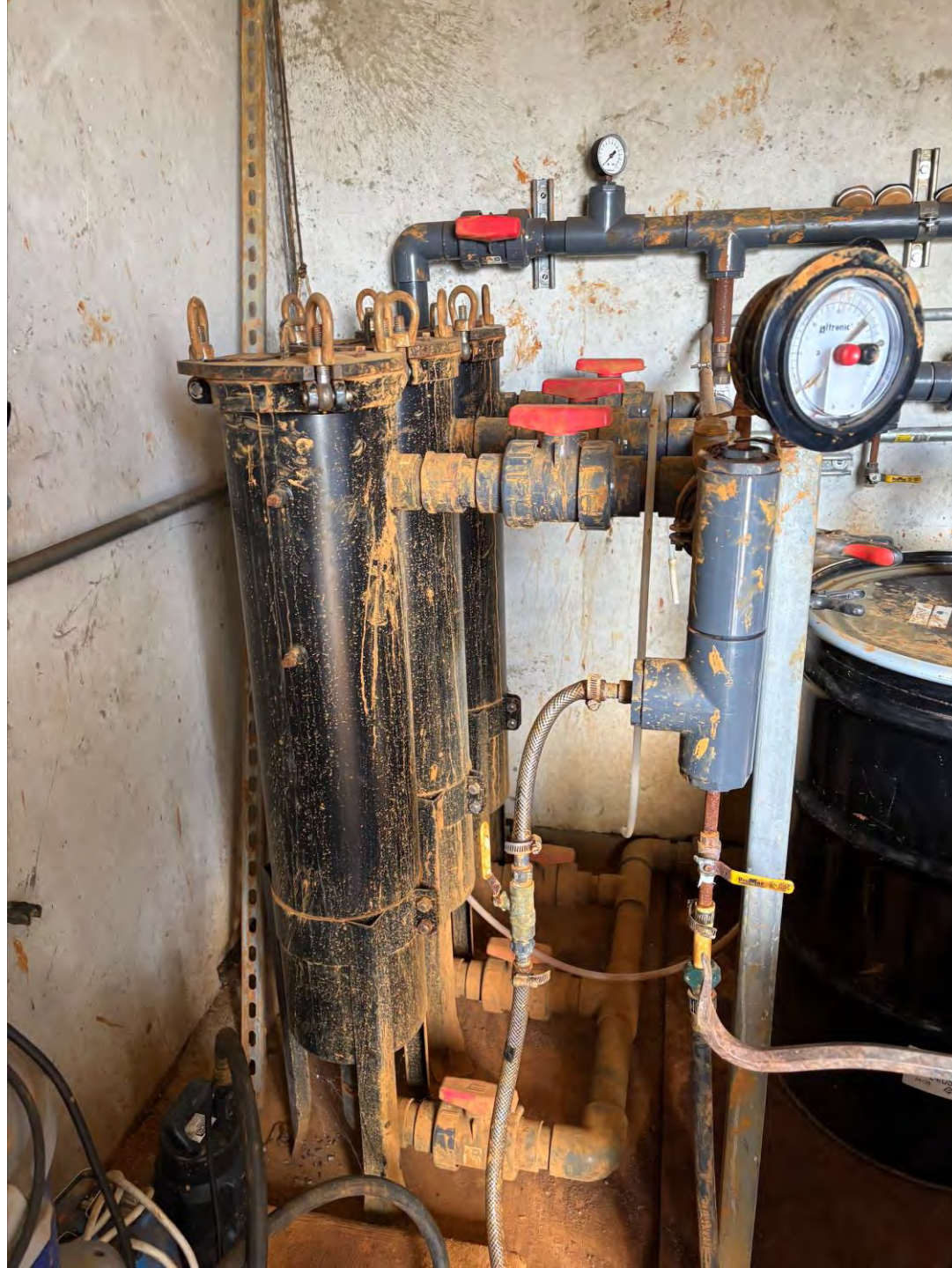
Inside the pump building
