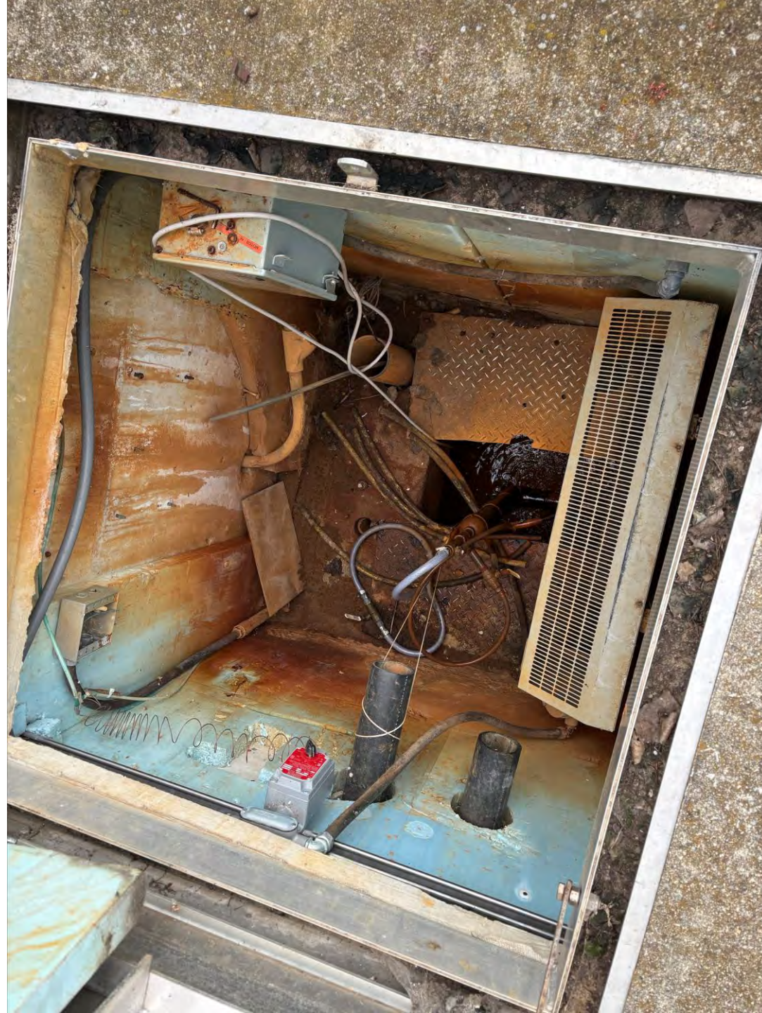
Groundwater well with heater
