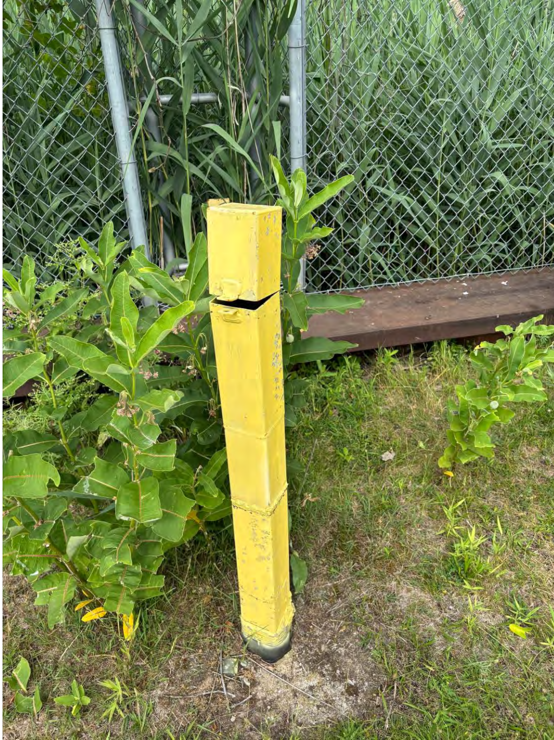
Unmarked, unlocked and open well
