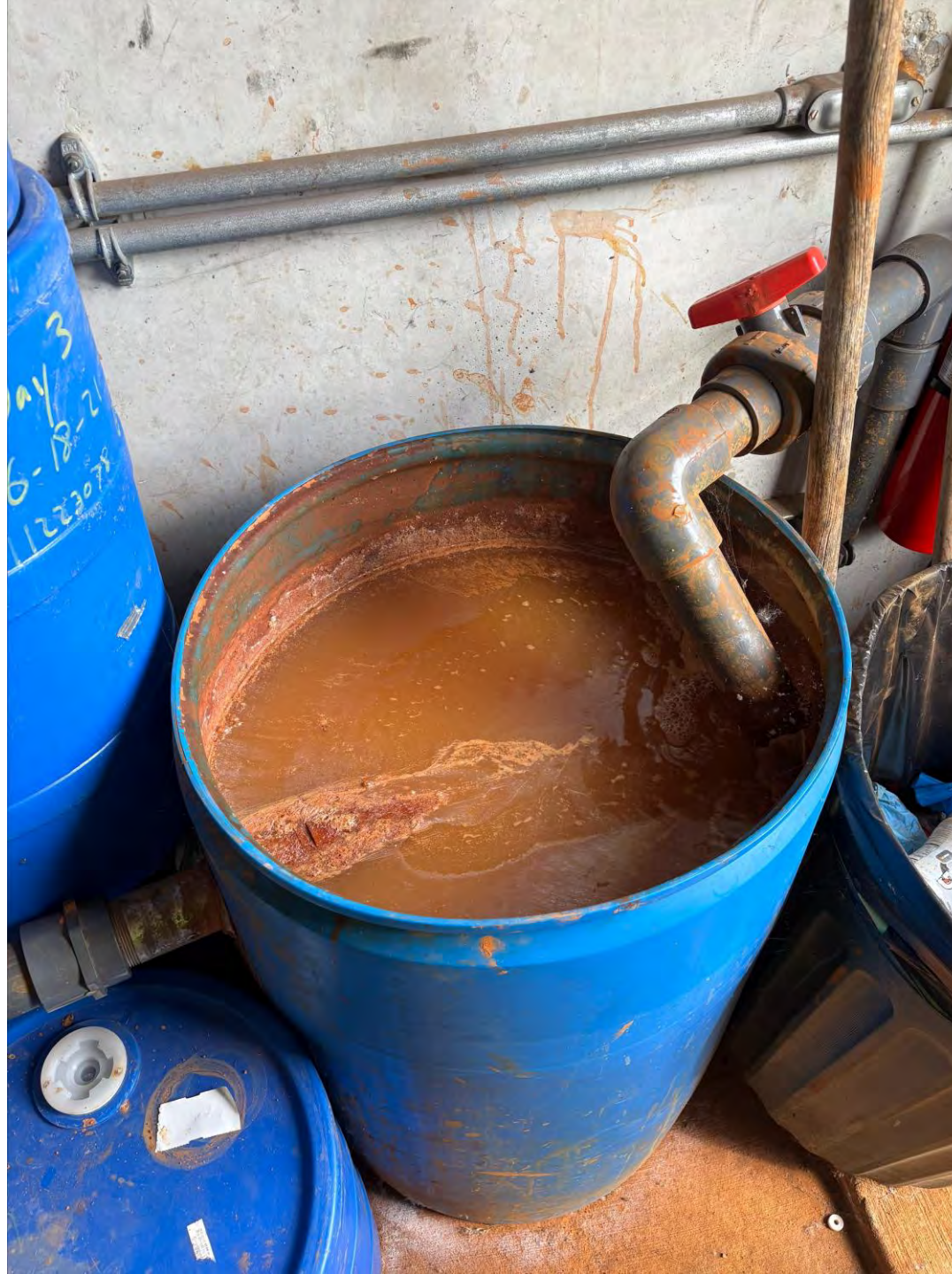
Inside the pump building
