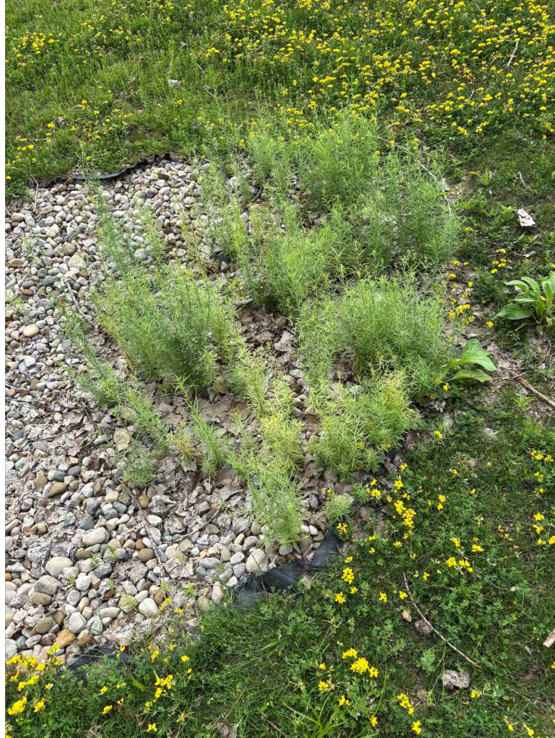
Long vegetation growing in the gravel ditch
