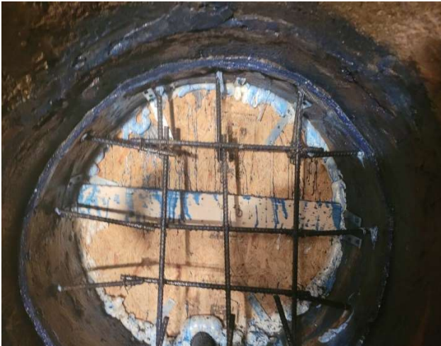
Viewing form, rebar with water stop and flow through pipe from the front. Front side of form to be installed.
