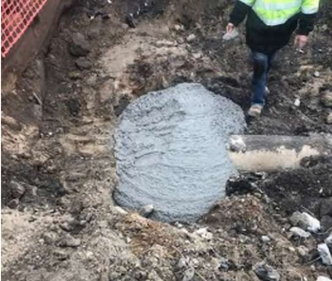
Filled remaining section of pipe and disconnect void with concrete prior to backfilling.
