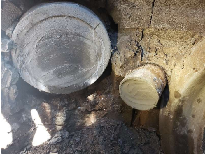
Two sealed lateral plug locations prior to a disconnect.
