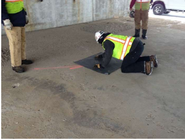
Example of lining installed under manhole cover, secured with silicone. Manhole cover reinstalled over lining.
