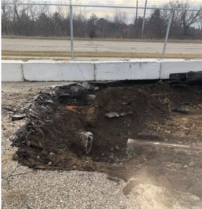
Example of disconnect in line. Sewer line excavated, disconnected, temporarily plugged prior to sealing.
