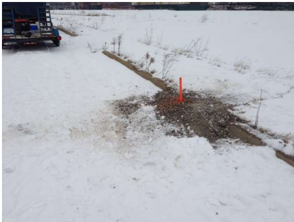
Example of steel plate then covered in gravel mound and marked for visibility.
