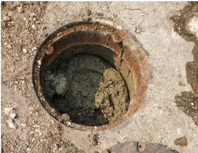
Partially full manhole with concrete, small pours conducted to streamline elimination of voids at smaller increments.
