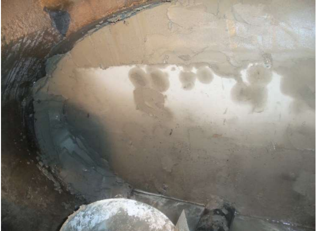
Example of grouted, sealed concrete with form removed. Flow through pipe still in place while additional curing occurs.
