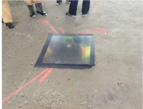
Example of additional silicone applied over manhole, another liner installed, then covered with steel plate.
