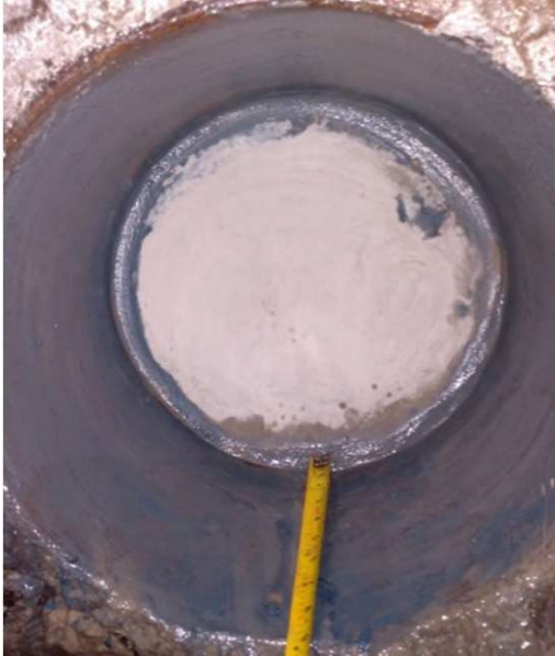
Plug with additional bonding agent applied after adding grout and water stop
