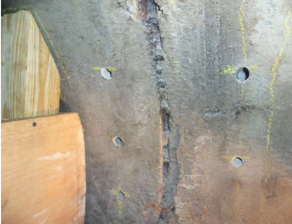
Example of rebar support preparation with bulkhead back form frame to left.
