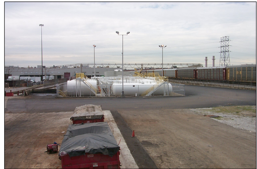
VIEW FACING SOUTH, WITH CHIP PAD IN THE FOREGROUND AND MORaine ENGINE TANK FARM IN THE BACKGROUND.
