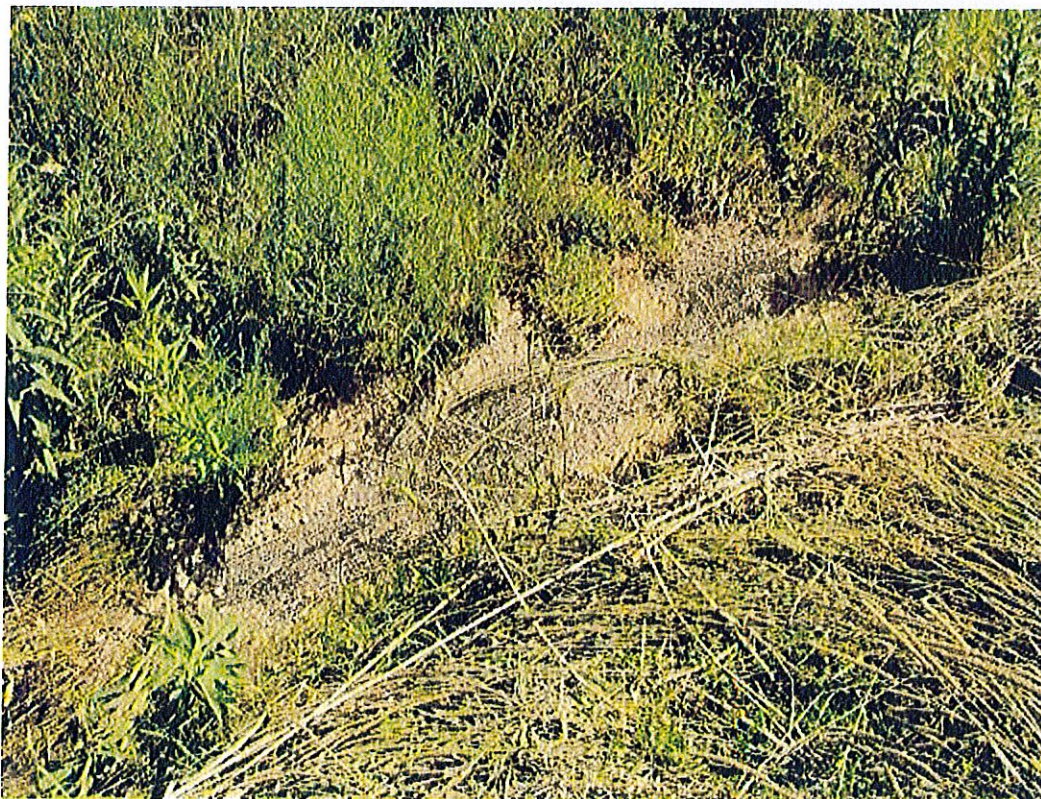
Photograph 20: Exposed geotextile fabric due to erosion along CB-3 overflow spillway.
