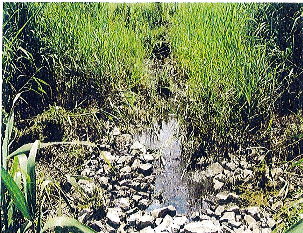
Photograph 18: CB-3 partially clogged.
