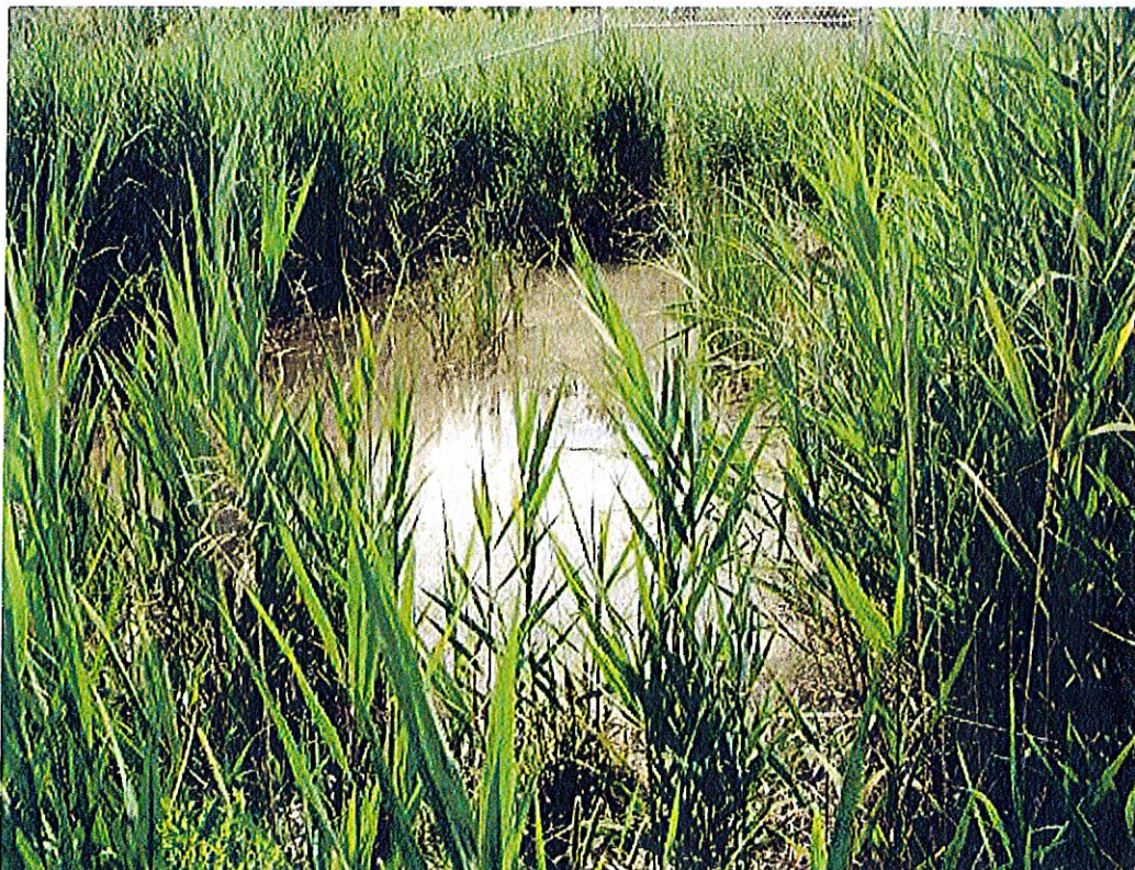
Photograph 14: Stagnant water in CB-2 indicates clogging.
