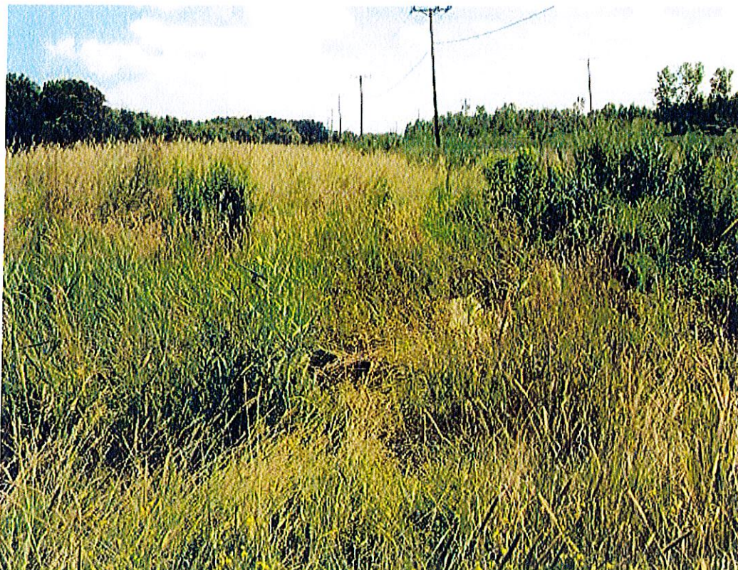
Photograph 7: View looking east of CB-1 overflow spillway showing significant vegetation.
