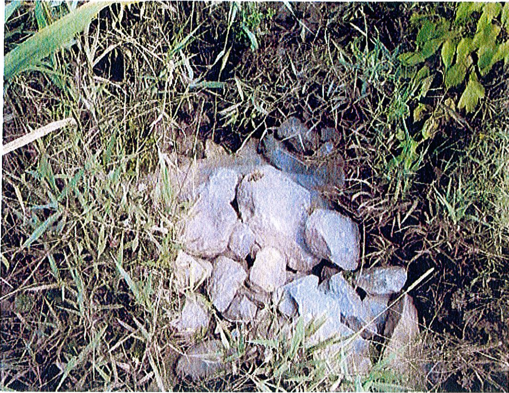
Photograph 9: Woven geotextile exposed due to erosion where CB-1 overflow spillway crosses access road.
