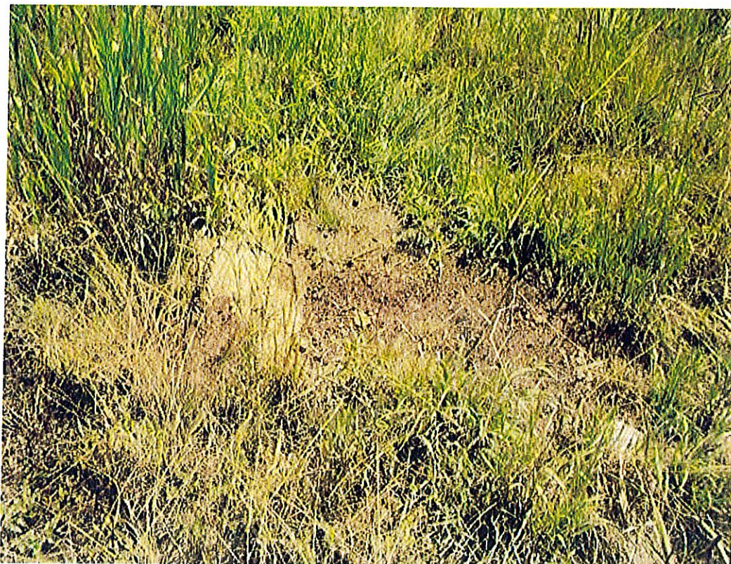
Photograph 15: View of soil with no vegetation in CB-2 overflow spillway near access road.
