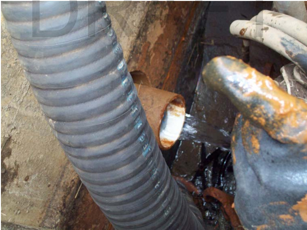
Photo 4: North west side of pump station prior to plug with water flowing from pipe.
