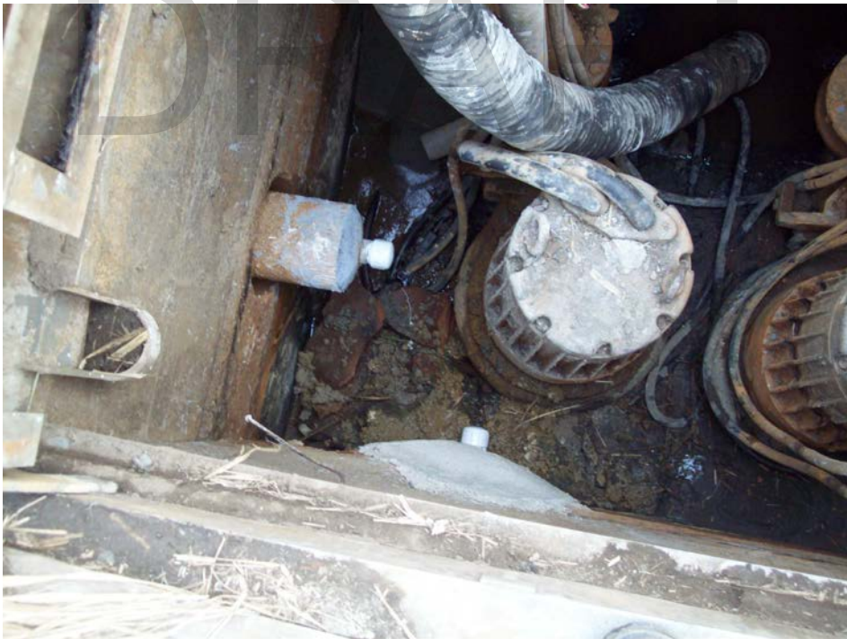
Photo 8: West side of pump station piped plugged and capped.
