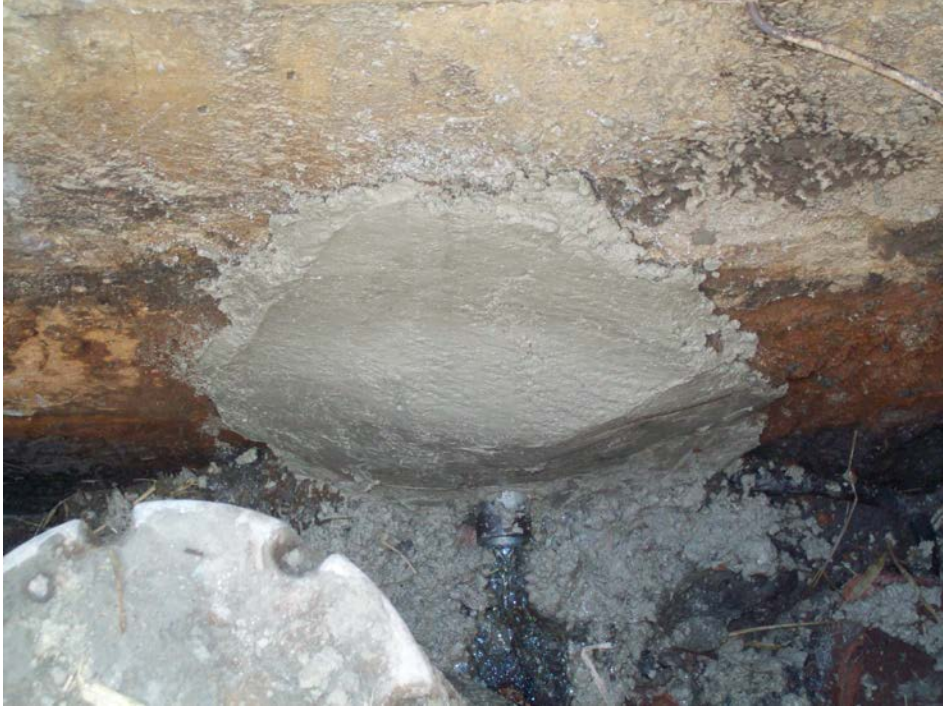
Photo 7: West side of pump station pipe plugged
