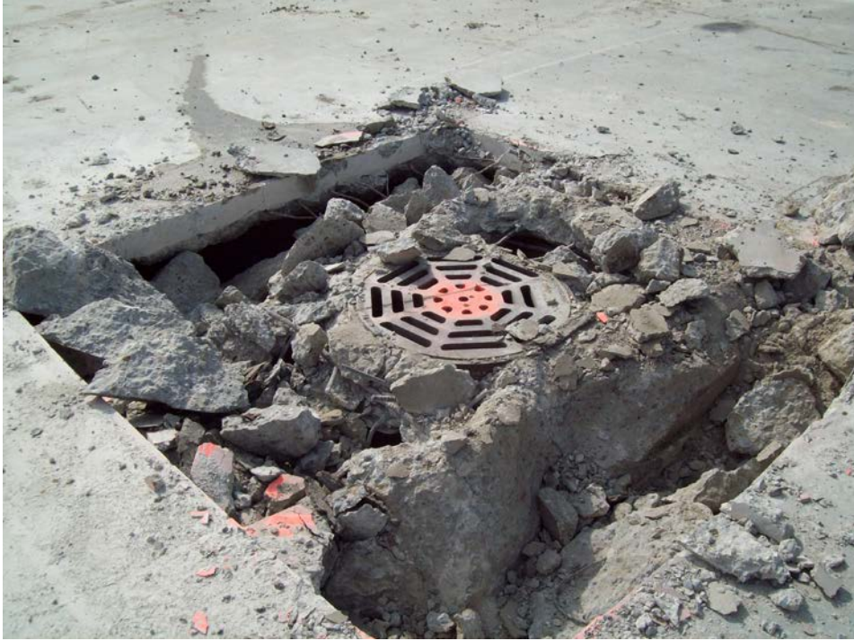
Photo 5: Storm sewer inlet to be capped is rectangular shape.
