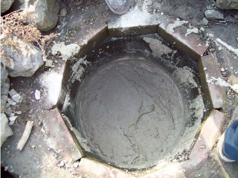
Photo 19: Filled in catch basin at corner of Montcalm and Saginaw
