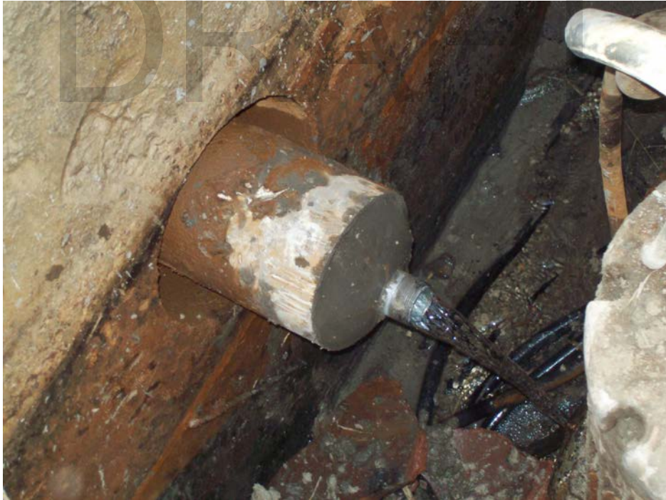
Photo 6: North west side of pump station pipe plugged.
