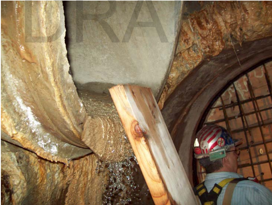
Photo 16: Water coming into ST8A from a pipe on the east side of the storm main.
