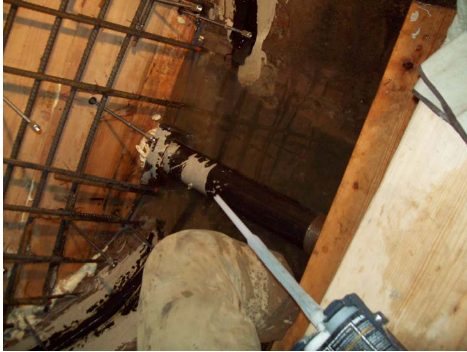
Photo 13: Form inside ST8A
