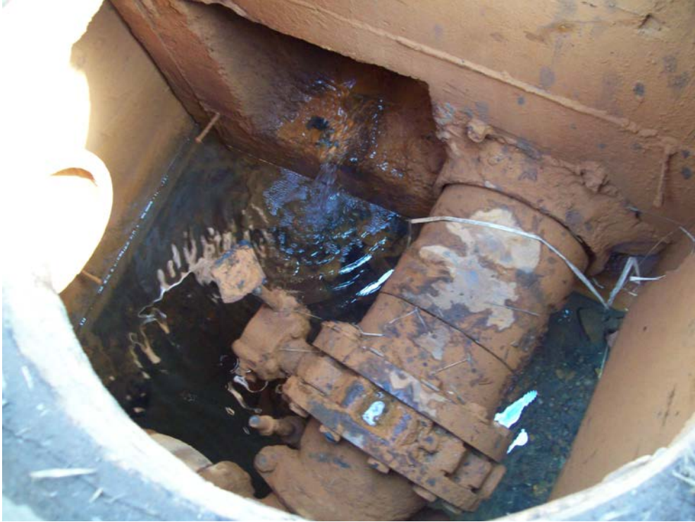
Photo 3: North east side of pump station prior to plugs. Water flowing from pipe.
