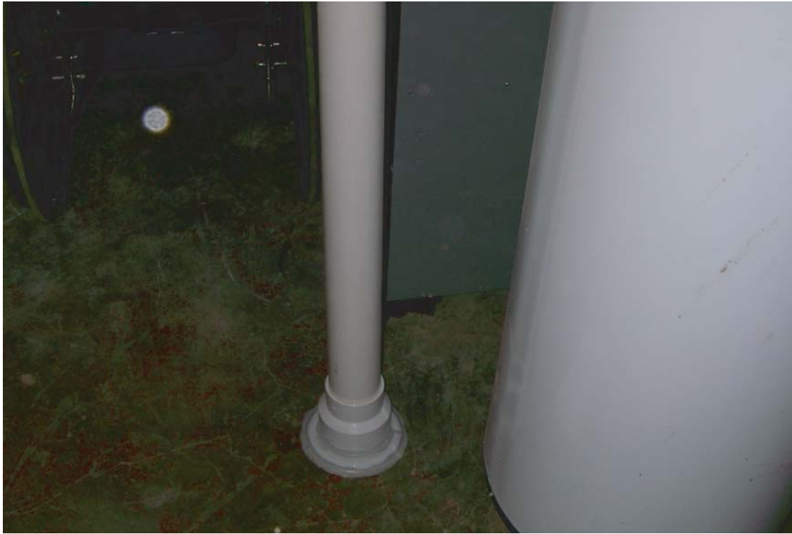
PHOTOGRAPH 3: Extraction point. PVC piping extends through the concrete slab floor or crawl-space liner. PVC pipe extends upward to an overhead piping system routed to an “in-line” fan or turbine used to vent the sub-slab space.
