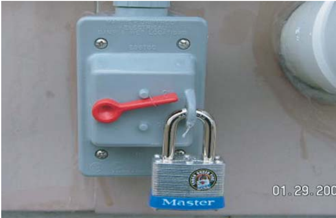
PHOTOGRAPH 9: Padlock located on the “on/off” switch located on the exterior of your structure. This system is designed to run in the “on” position at all times to ensure it is effective.
