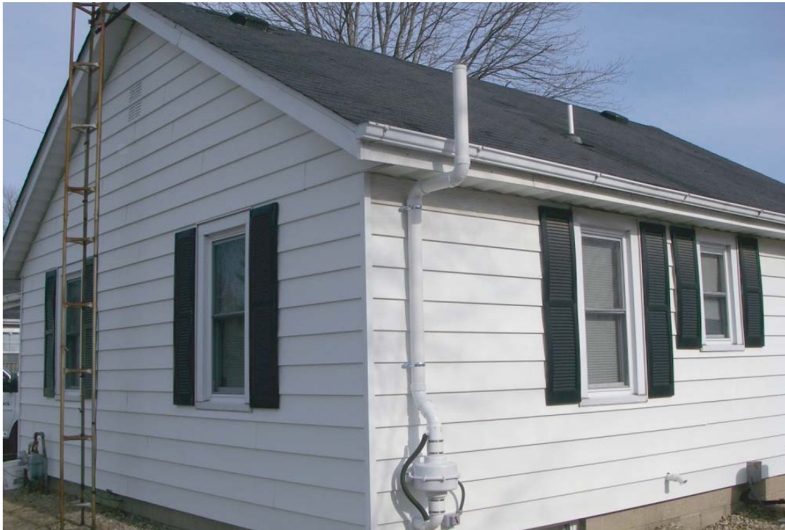
PHOTOGRAPH 1: Mitigation system fan and discharge. The fan creates a vacuum under the concrete floor slab or crawlspace. The vacuum draws vapors from under your home into a PVC pipe system that is vented above the structure. The fan must be “on” and running 24 hours a day to ensure the system is operating effectively. The vent pipe must be clear of obstructions at all times. This includes caps and covers.
