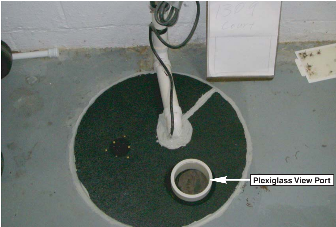
PHOTOGRAPH 7: Sump cover installed and sealed. Lid view port can be used for pump performance inspection without lid removal.
