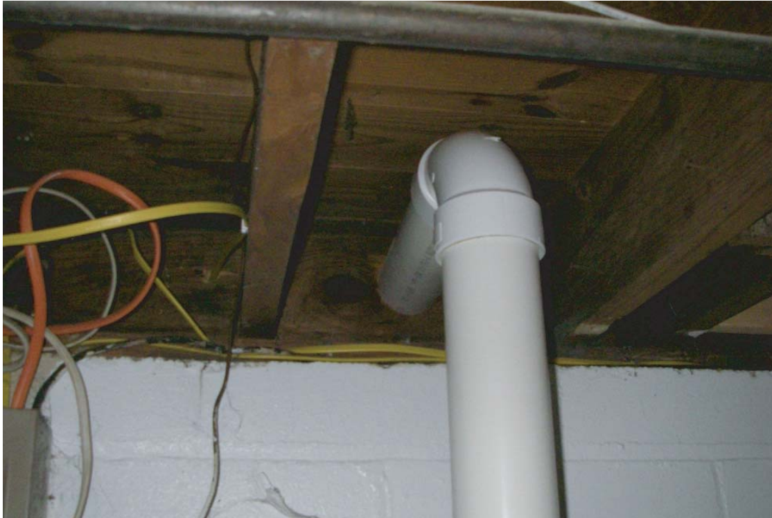
PHOTOGRAPH 4: Overhead extraction piping to exterior fan or turbine. Horizontal piping is installed at a 1% slope back the extraction point. Pipe is supported every 8 feet on vertical piping, every 6 feet on horizontal piping, and near the discharge.
