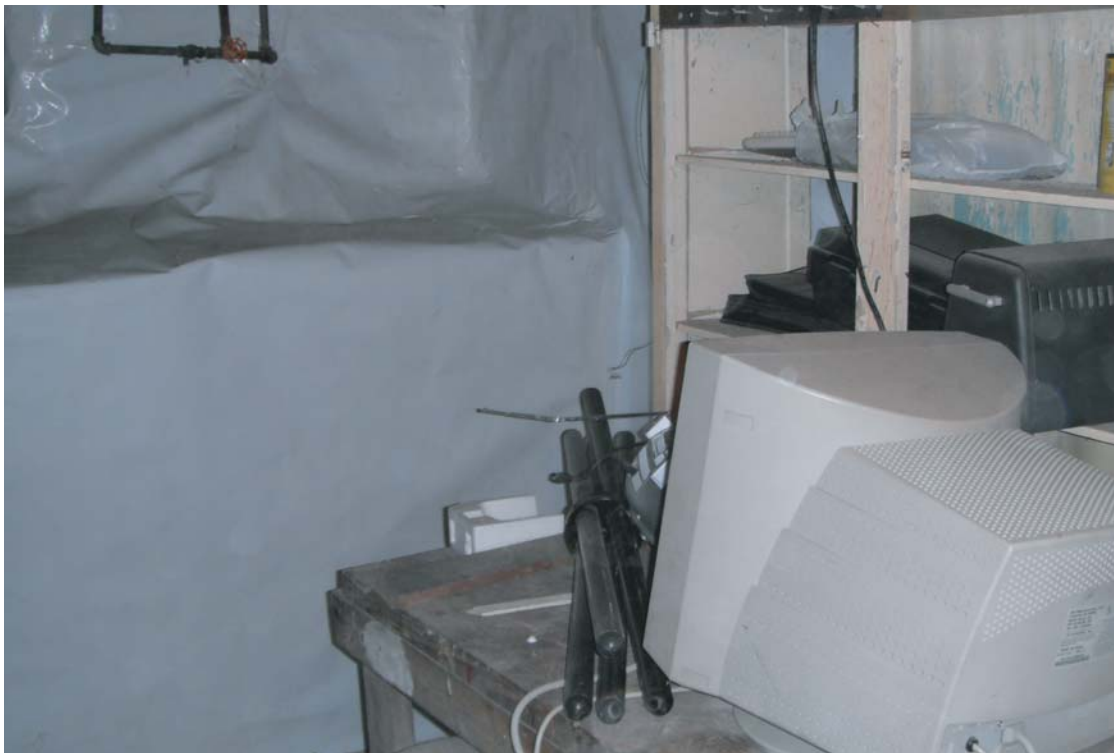
PHOTOGRAPH 6: Liner used to seal damaged wall. Liner should be maintained to ensure vapors are captured by the mitigation system.
