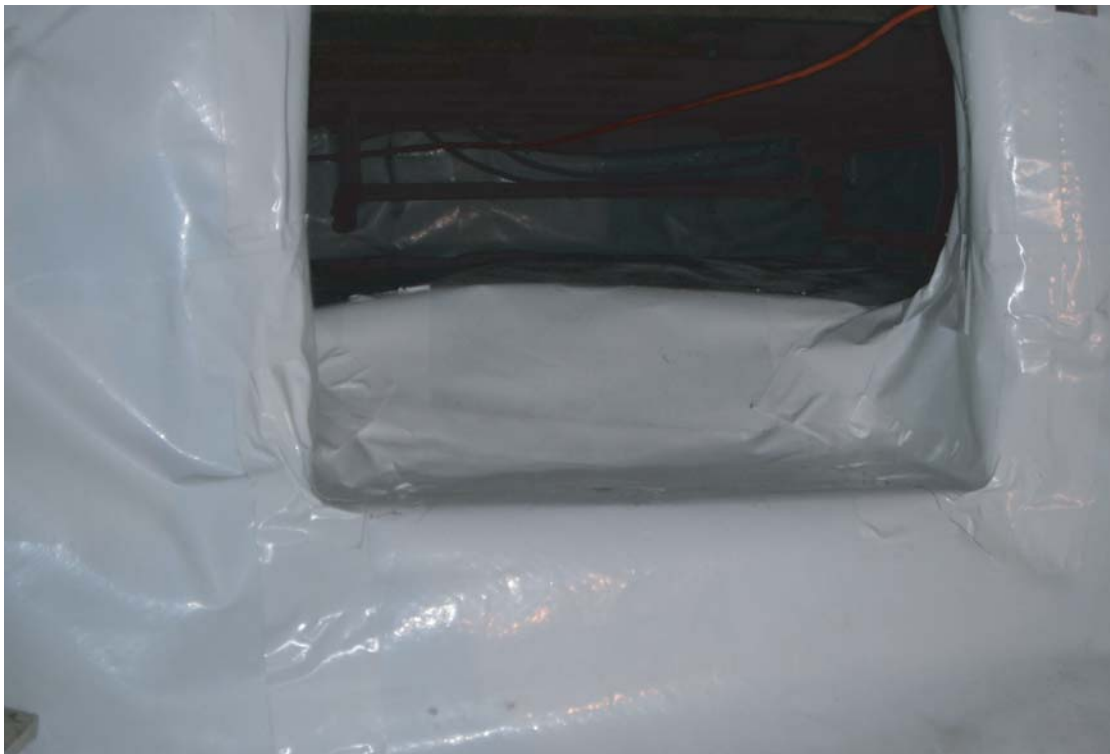
PHOTOGRAPH 8: Crawlspace sealed using polyethylene sheeting. Sheeting is sealed at the perimeter of the crawlspace and around any protrusions. Polyethylene sheeting installed in areas accessible to foot traffic or used for storage are protected using foam padding and untreated plywood.
