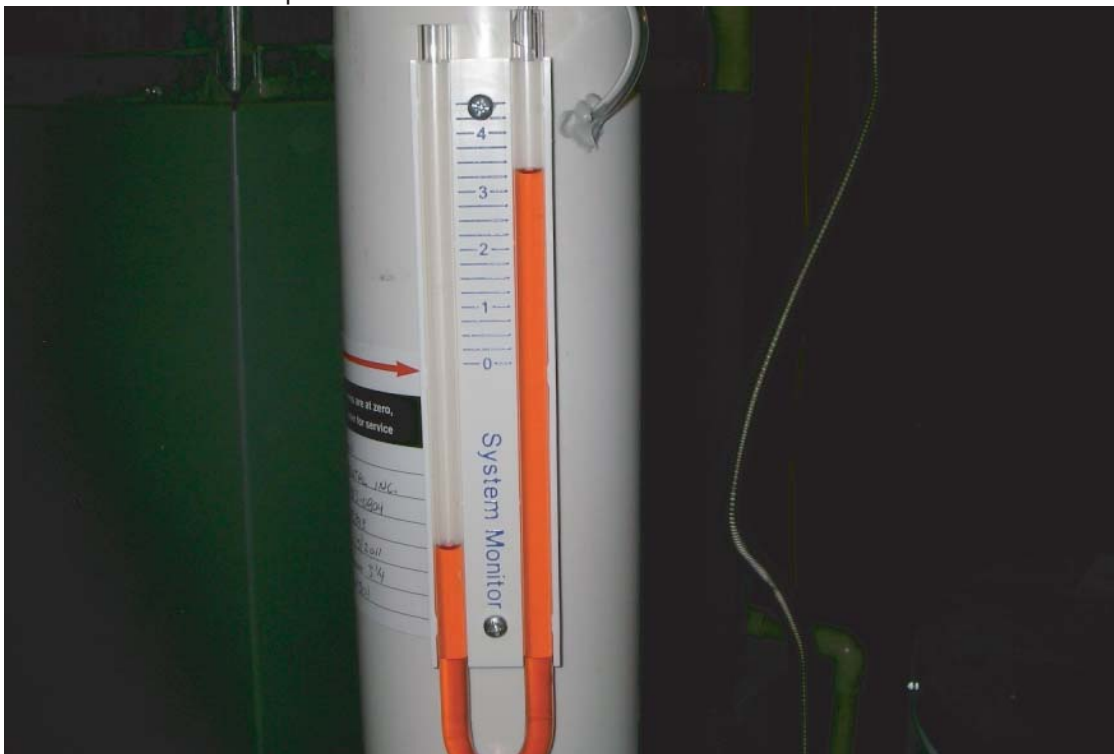
PHOTOGRAPH 2: Manometer (vacuum pressure gauge) to monitor system performance; the “u-tube” will display a reading greater than zero (the system is designed to operate between 1-4 inches of water column) on the side where the small poly tubing is located when the system is operating effectively.
