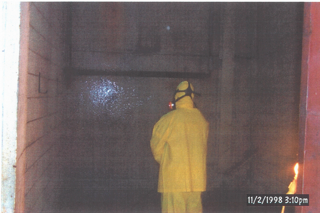
Nodular Iron Oil House, RCRA Storage Unit Steam Cleaning After Scrubbing (Viewing South)
