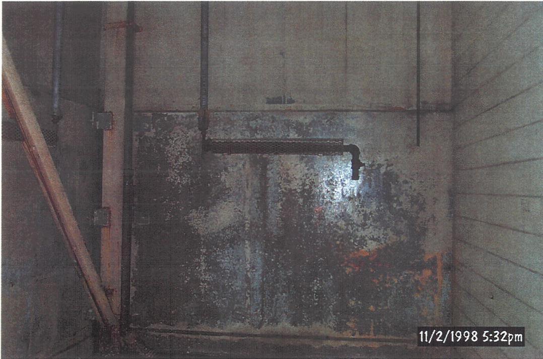
Nodular Iron Oil House, Inside RCRA Storage Unit (Viewing South After Final Cleaning)
