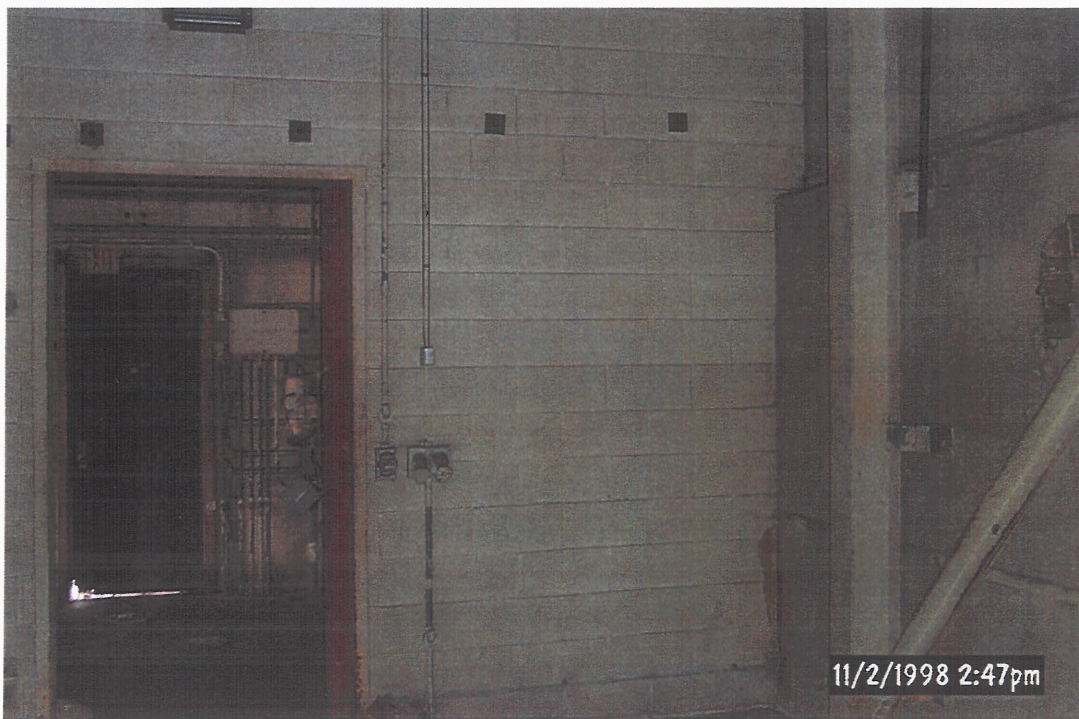
Nodular Iron Oil House, Inside RCRA Storage Unit (Viewing North - Prior to Cleaning Activities)
