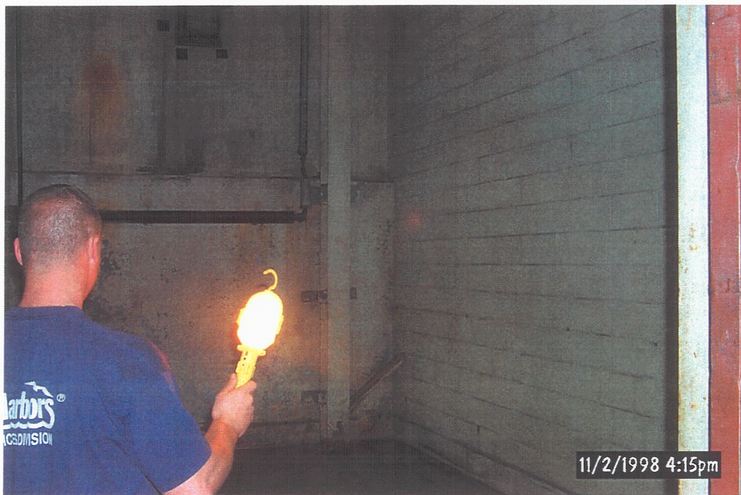
Nodular Iron Oil House, RCRA Storage Unit After Steam Cleaning Activities (Viewing South)
