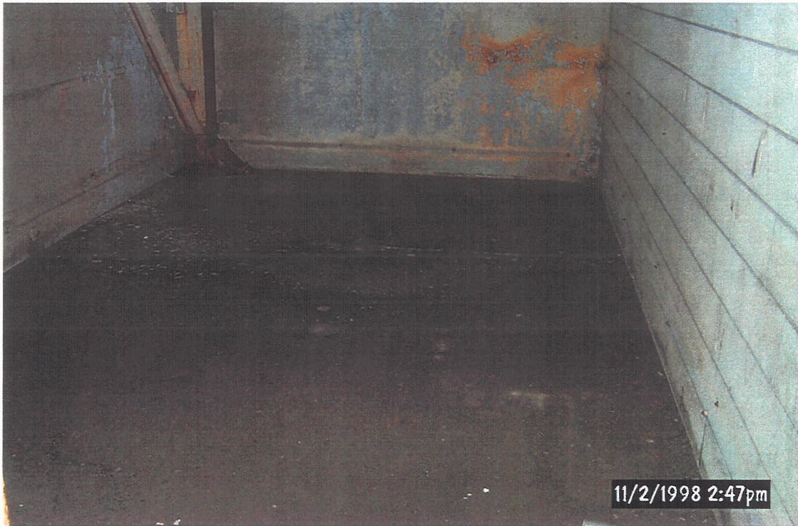
Nodular Iron Oil House, RCRA Storage Unit (Viewing South - Prior to Cleaning Activities)
